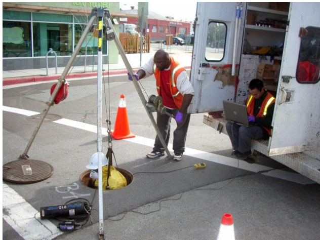
Flow Monitor Installation for the City of Berkeley
